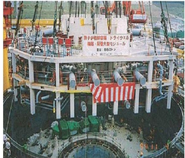
Installing The Upper Drywell Super Large Scale Module At Kashiwazaki Kariwa-7 In Japan:
